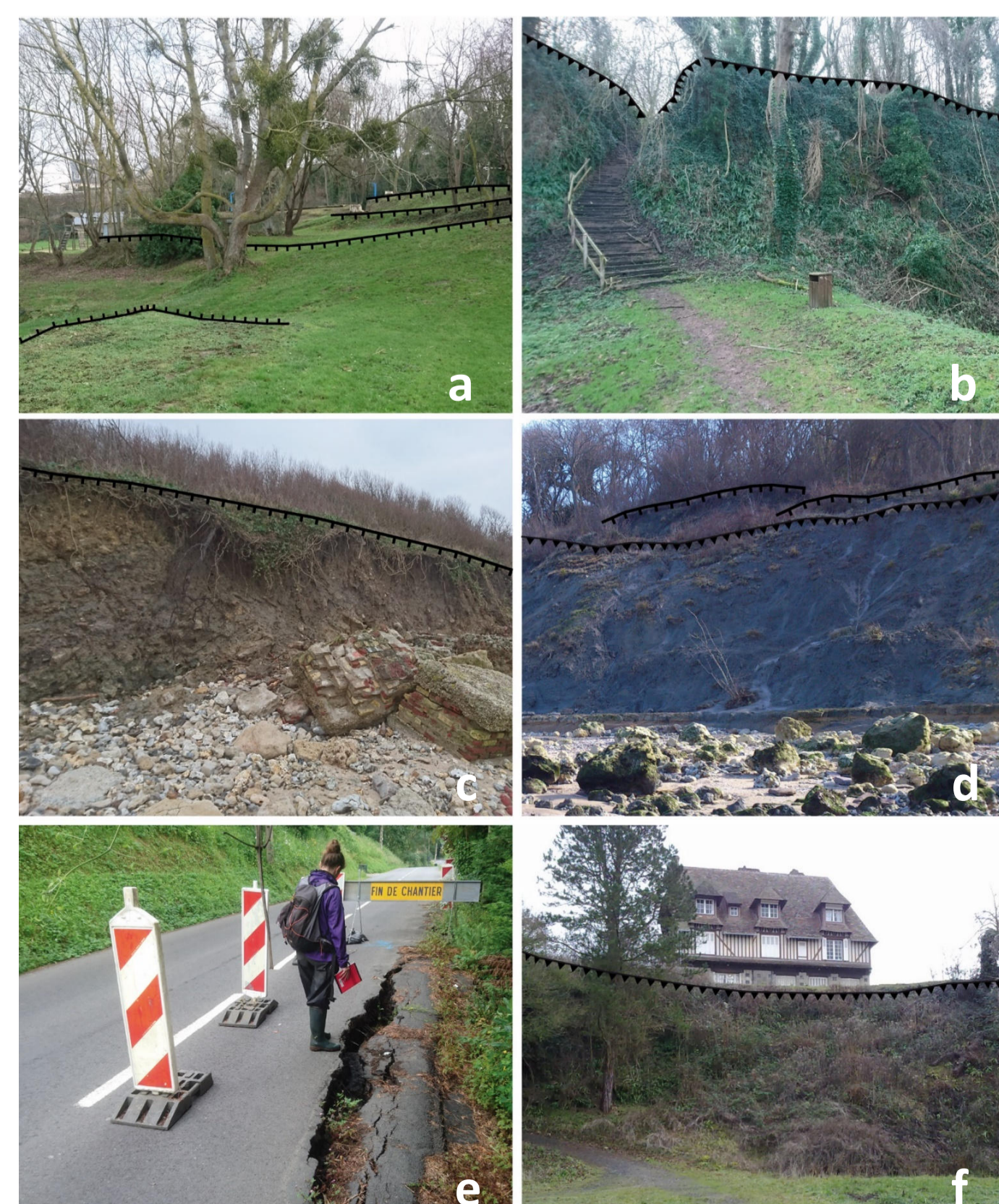
Fig. 6 - Main geomorphological features encountered in the Cirque des Graves (location given in Fig. 4). (a) Minor scarps and stairs morphology; (b) Main scarp of the cirque (chalk outcrop); (c) Heads (reworked formations) at the foot of the landslide; (d) Mudflows in Oxfordian marls on the coastline; (e) Recent crack on the RD513; (f) Building near a major scarp in the middle of the slide
