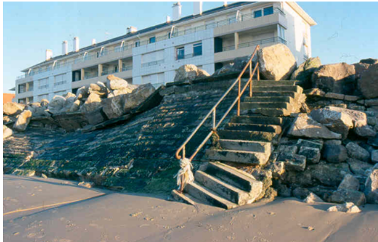
Figure 1.7. Lowering of the beach at the foot of a structure, Wissant, France (source: C. Meur-Ferec, 2003). For a color version of this figure, see www.iste.co.uk/rebotier/risks.zip
