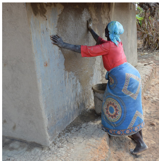
Women are involved in the construction, maintenance and protection of houses against particular hazards. Houses become more resilient thanks to this knowledge and know-how. Woman plastering in Chisi, Nzimba. © Jon Twingi
