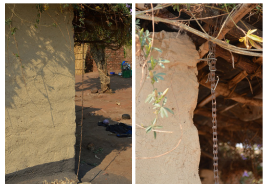
The roof structure is fastened to the ground with a motorcycle chain, what provides an additional connexion thus preventing the roof from being entirely blown off under wind pressure. House in Nsangu, Salima. © Jon Twingi
