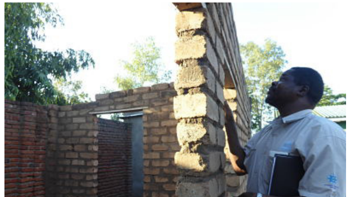
Walls with insufficient thickness and an important height are dangerous in the events of a disaster as they are not stable enough. CC- Ignasio Ngoma
