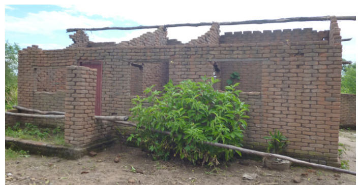
CGI sheets roofs can easily be blown off at high speeds in the event of strong winds creating an important risk. When the roof of the veranda is not separate from the roof of the main structure, the uplift of the entire roof can more easily happen. House in Karonga. © Sonia Molina
