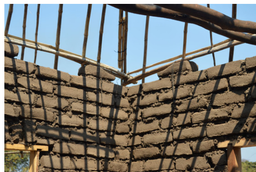
The roof structure is tied to the wall through several wrappings of galvanised metal wire, avoiding to wrap the metal wire in correspondence to vertical mortar joints. House under construction in Chakwela, Mangochi. © Jon Twingi
