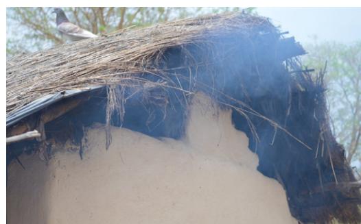
Kitchens always present openings to let the smoke out. Smoke has very bad impacts on people's health, but at the same time it treats thatch against insect attacks: Thatched roofs let the smoke out more easily as they are porous (William, Rumphu). © Jon Twingi
