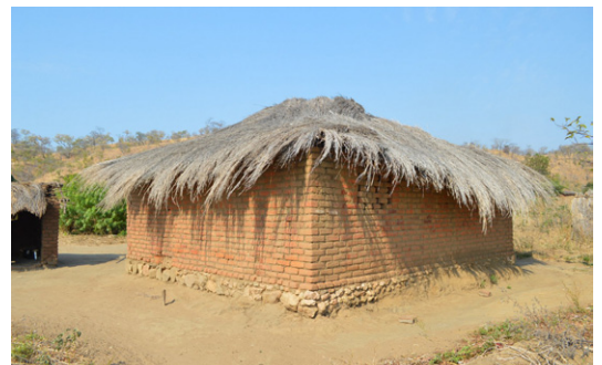
Stone foundation and plinth (Chimwendo, Karonga) protecting the walls from humidity and floods. © Jon Twingi.
