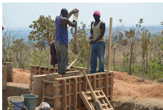
Many constructions in Malawi are built using local, renewable materials with little impact in the environment when they are well managed. This image shows the construction of a rammed earth house in Nisanje, Lilongwe. © Jon Twingi
