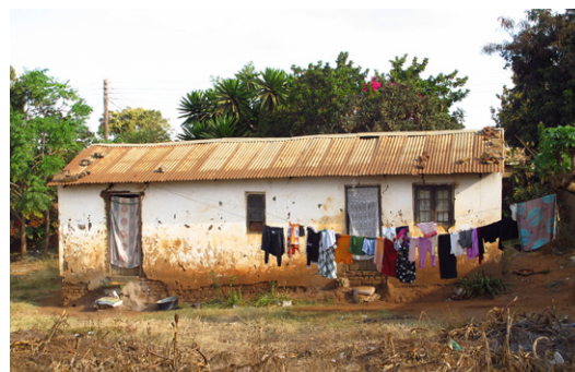
These two houses would be semi-permanent according to different authors as they are built with a mix of materials. The one on top has burnt bricks and thatched roof (Kachopatsonga, Nkhata Bay- © Jon Twingi). The other one has adobe brick walls and metallic roof (Lilongwe- © Urbanopolista)
