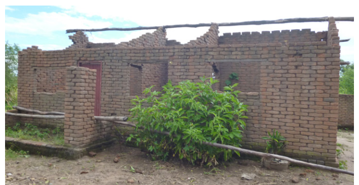
CGI sheets roofs can easily be blown off at high speeds in the event of strong winds creating an important risk. When the roof of the veranda is not separate from the roof of the main structure, the uplift of the entire roof can more easily happen. House in Karonga. © Sonia Molina
