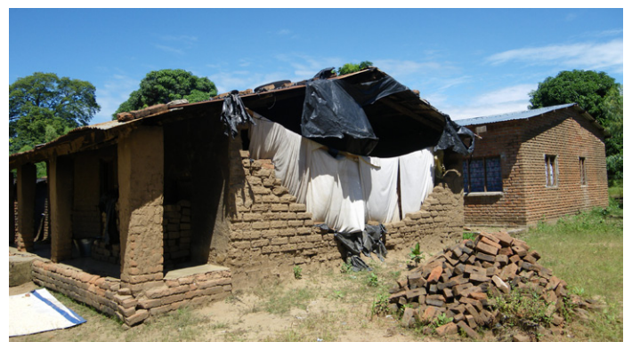
Unsupported masonry gables tend to fail in the out-of-plane direction in the event of an earthquake. This house's gable fell after the Karonga earthquake in 2009. © Sonia Molina
