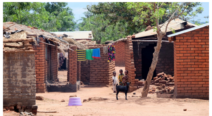
Constructions with various dangerous elements such as disconnected masonry columns and very thin and high masonry walls. CC- Ploughmann
