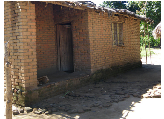
Raising dampness creates unhealthy living conditions inside the houses due to moisture. © Sonia Molina
