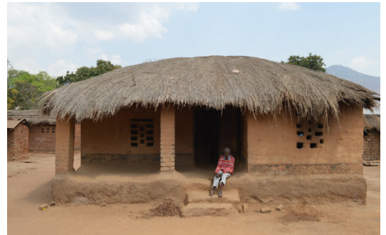
Houses constructed using adobe bricks, render and earth mortar like this one (Chisoka, Rumph District) responded well to the important floods in 2015 (CRS, 2020) as the design developed over centuries provides protection from the elements. Other than some minor repairs, some of these houses were in good condition and allowed the families to return to their homes once the floods had subsided. © Jon Twingi
