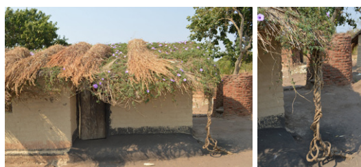
In some villages, the roof is used as a support for climbing plants. The risk of wrenching as well as partial or total uplift is reduced as the plants fasten together the roof components and attach the roof to the ground through the roots. House in Nsangu, Salima. © Jon Twingi
