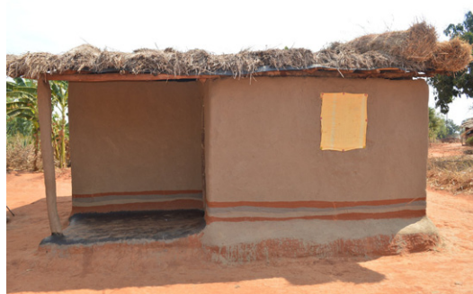
Thatched roofs are repaired when necessary. This house in Chome (Rumphi) presents thatch bundles which can be easily replaced when they get rotten. © Jon Twingi
