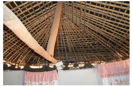
Bamboo is more and more used, for example in roof frameworks. Hipped roof in Dzipusile, Ntcheu. © Jon Twingi.
