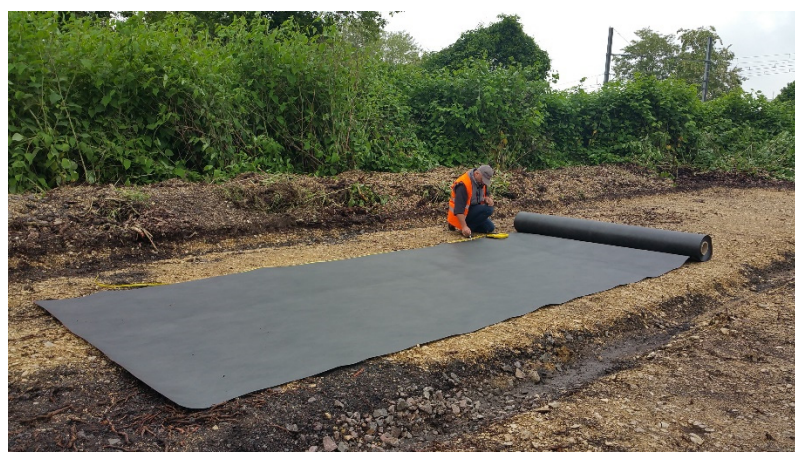
Figure 1. Installation of a synthetic geotextile as part of a tarping operation to control Asian knotweed. © INRAE.
