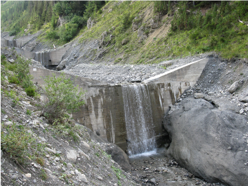
Figure 1. Series of check dams. Saint Antoine torrent, Modane, France, 2014 (Source: INRAE, ETNA team).
