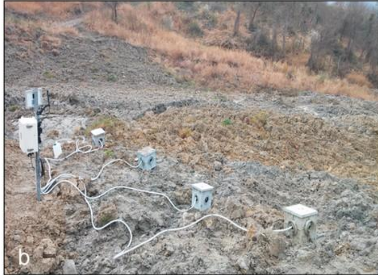
Fig. 9: Example of a monitoring installation on the Montevecchio earthflow, where non-negligible relative displacement of the four seismic sensors might occur. From (Bertello et al., 2018).
