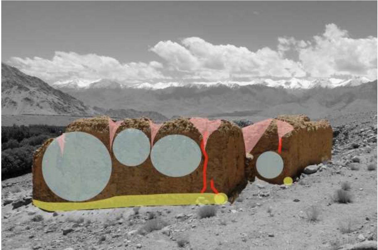
Fig. 22: pathologies on the outer side of the northern wall, temple Co1, Leh Choskor. ©MAFIL/Sadozai.
