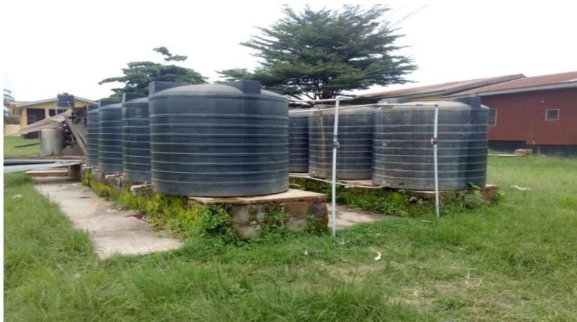
One of the water distribution outlets of gofamint. Credit: tobe nneli
