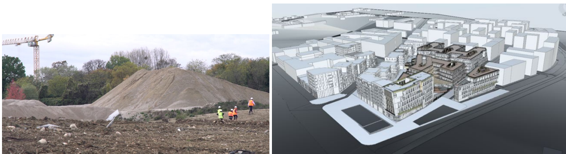
Figure 2. LaVallée: a 500 m × 400 m urban district under construction at present. Right: digital models of the buildings to be built.
