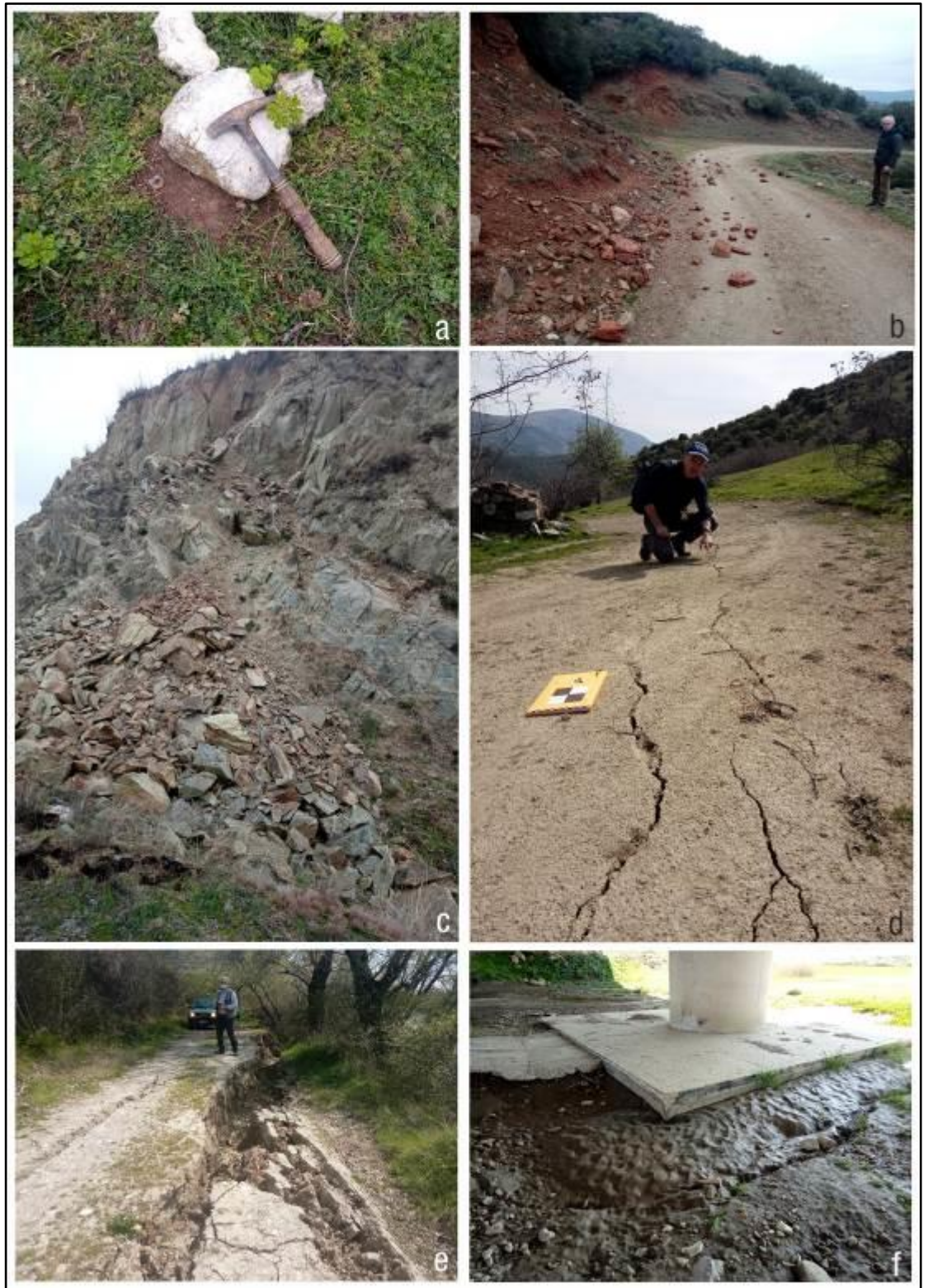
Fig. 12: Field photographs showing a) Uptrown rocks in a gentle slope near Tsouma Monastery (Location 3 in Fig. 10) b) Rockfalls and debris along a mountainous road south of Damasi c) Rockfalls and wedge chips in a road cut north of Grizano d) Tension cracks north of Zarko, possibly along the surface projection of the M6.3 rupture plane (Location 4 in Fig. 10) e) Lateral spreading phenomena along the Pinios river valley, north of Koutsochero. f) Liquefaction at the base of the bridge pillars. Larissa – Trikala new highway bridge over Pinios river, west of Koutsochero (location 5 in Fig. 10).
