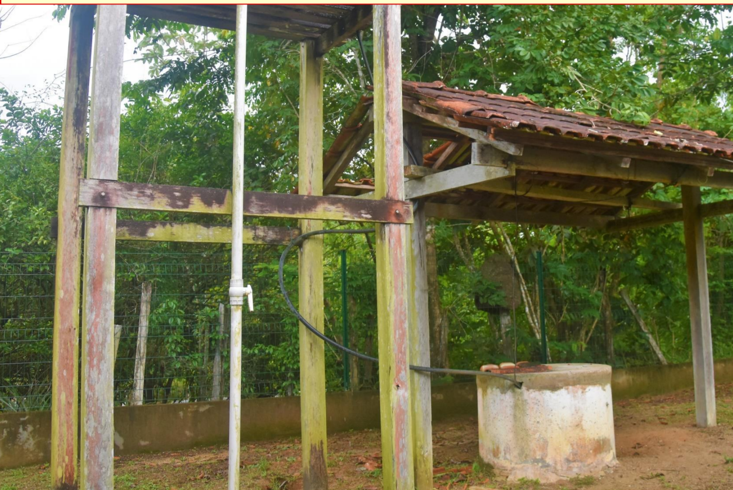
Fig. 3 : well n°4, a type of "Amazonian" well (dug), covered with cement and roof
