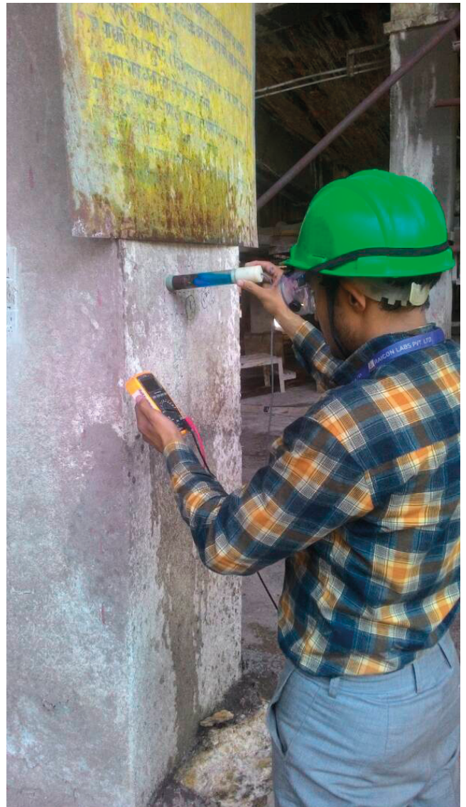
Figure 3. Half Cell Potential Test
