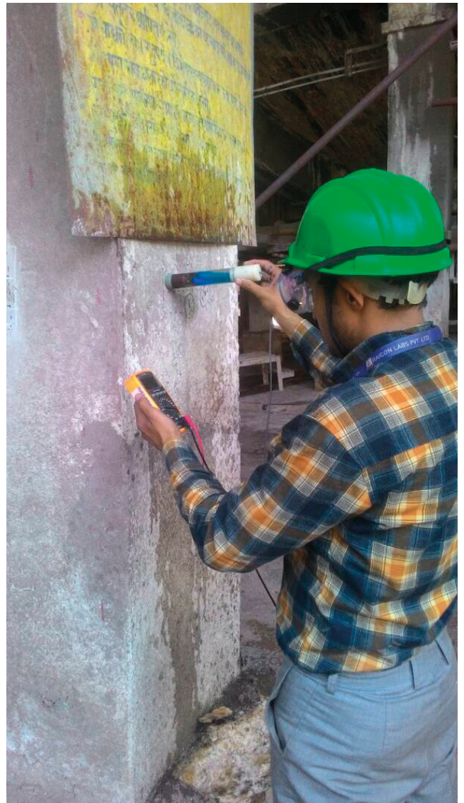
Figure 3. Half Cell Potential Test
