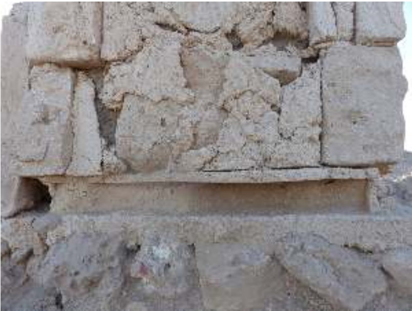
Fig 1-156 : moldings and prints visible in the groove, at the bottom of the pillar B12-05
