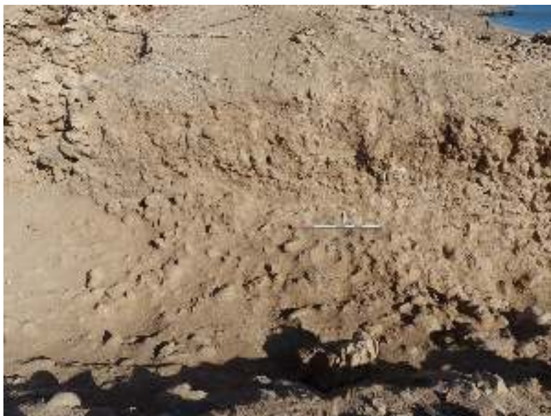
Fig 1-279 : the south wall B12-41 of the Mosque, badly preserved, emerging from the collapse in the south street
