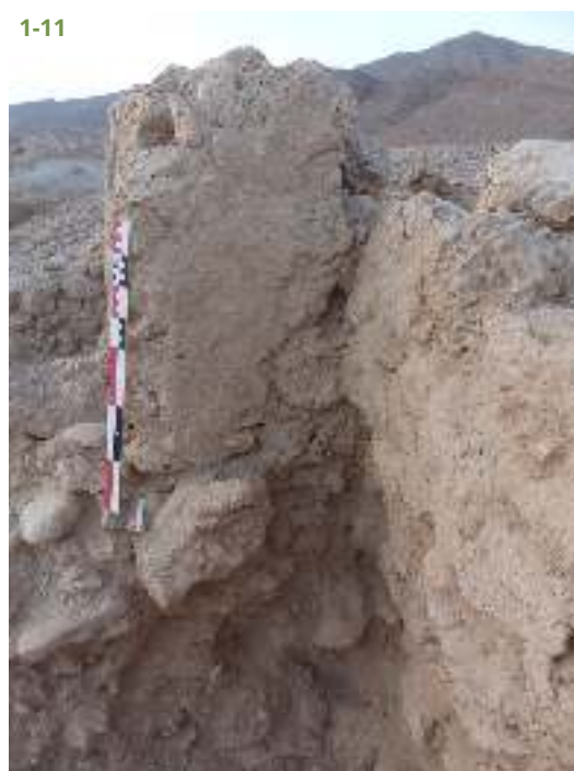
Fig 1-11 : the damaged buttress B12-321
