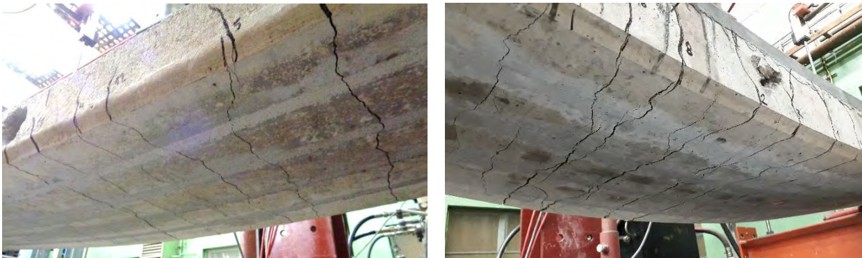
Fig. 4 Cracks at the bottom surface of the panels after executing experiments. Left figure is reference panel and right figure is panel with 30 mm UHPC.
