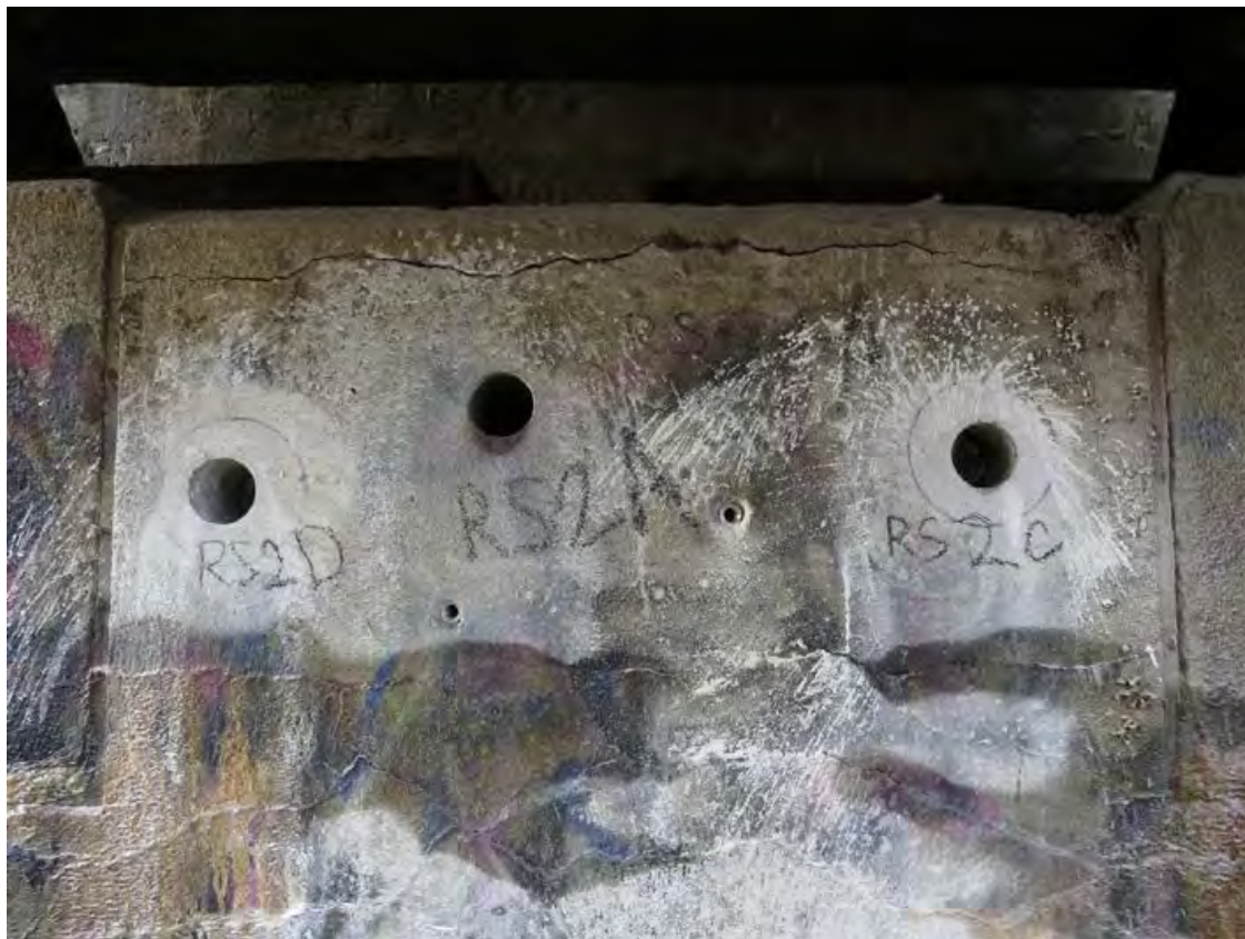
Fig. 2 The place where the specimens RS2-D, RS2-A, RS2-C were taken from the bridge abutment – a location with PRC (November 2019).
