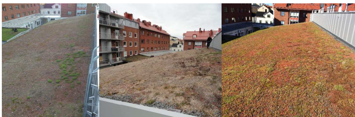
Figure 1: View of the same roof section. Left: end of May 2014, middle: early September 2014, right: early September 2015.
