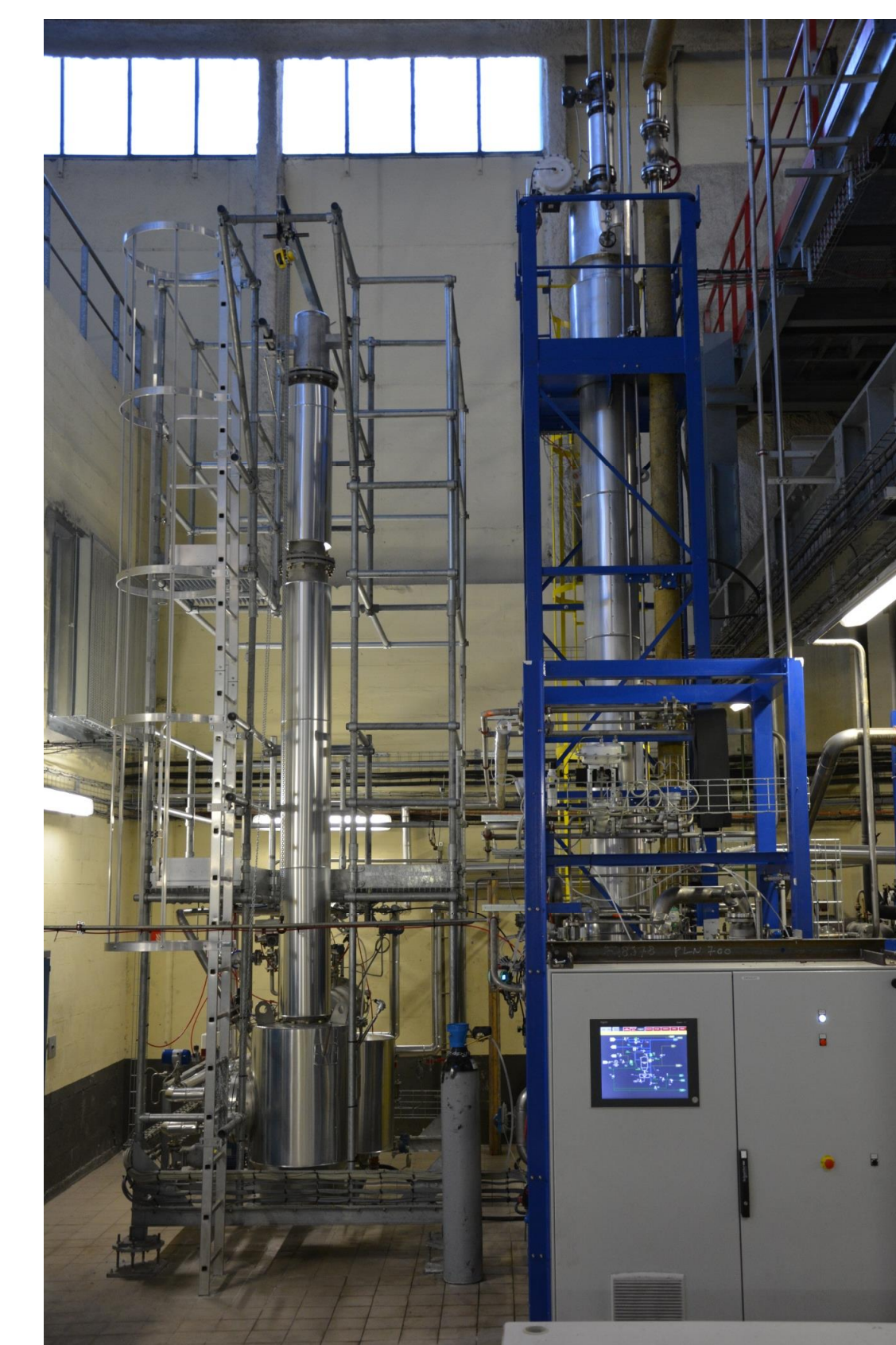
CO 2 -EnergiCapt demonstrator installed at the CPCU (LLT ®)
