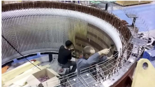
Photo: Jeumont Electric Precision Manufacturing: Workers build the stator of Ecoswing's onshore generator.
