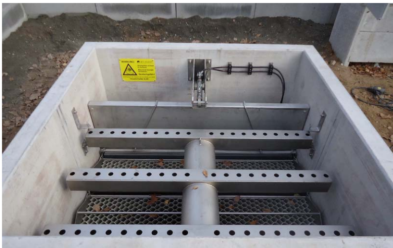
Fig. 10: Unit ready for operation (the overflow pipes with drainholes have been replaced by now by open gutters which are less sensitive to clogging by tree leaves)
