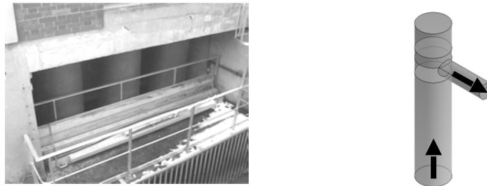
Figure 3: Photo of the three risers (left) - Model of one of the three pumps (right)
