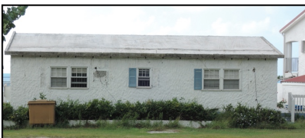
Figure 5. Concrete roof rebuilt after Hurricane Irma in Grand Case (Source: J. Gargani).
