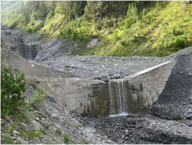
Figure 1 – Series of check dams located in the Saint Antoine torrent in France. Source: ©INRAE/ETNA, 2014.
