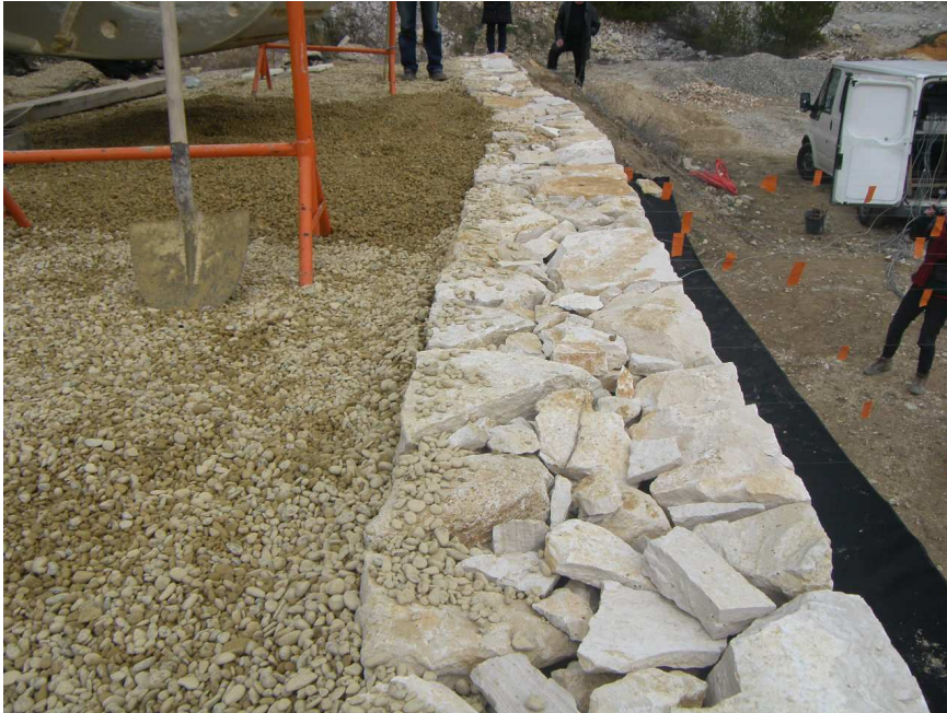
Figure 11. Deformation of the wall after stage 0.5III: top view.
