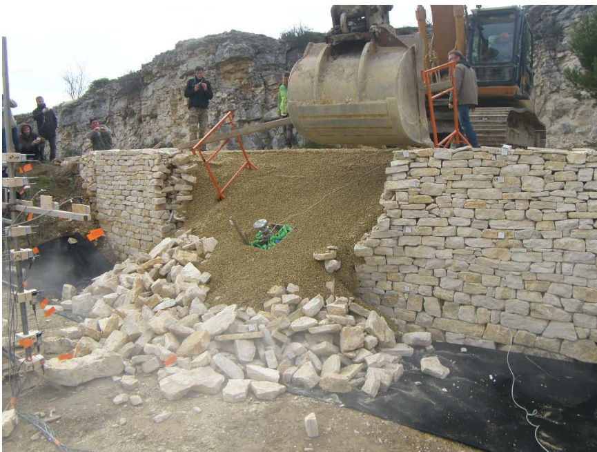
Figure 12. Test wall 2 after collapse.
