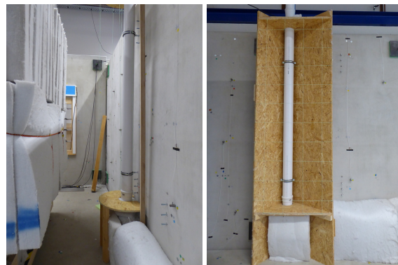
Figure 3: Left: Additional absorption opposite the pipe. Right: Asymmetrically positioned reflector behind the tube made from 25 mm OSB boards.
