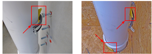
Figure 19: Detail of open clamps: Additional resilient material used to avoid contact with open clamp or OSB reflector.
