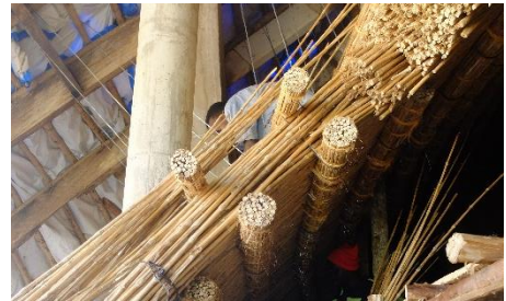
Section on the ceiling at the door level. Lower and upper rings are attached with binding wire
