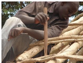
Workers sitting on the battens to work on the ceiling. Photo © Remigious Kigongo
