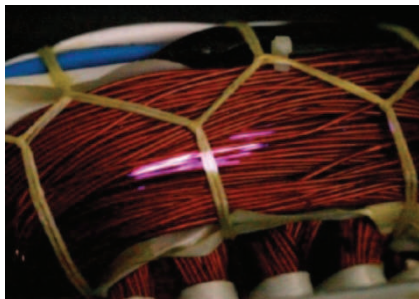
Fig. 2. Typical PD between neighbouring turns in a PWM fed motor[2]
