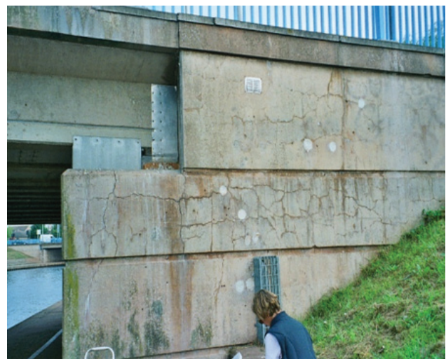
Figure 14 AAR damage from severe 2 mm/m to 4 mm/m variable expansions
