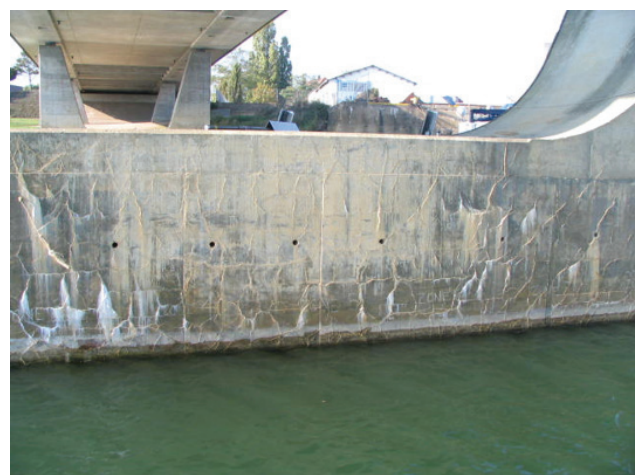
Figure 15 DEF damage from severe 1.5 to 5.5 mm/m variable expansions – (the white exsudations are calcite due to the dissolution of the lime of the cement and its carbonation with air)
