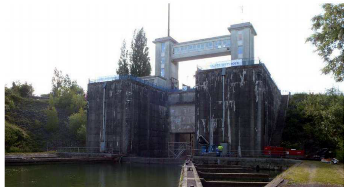
Illustration 2: Downstream part of the lock with the lower gate and its mask-girders.
