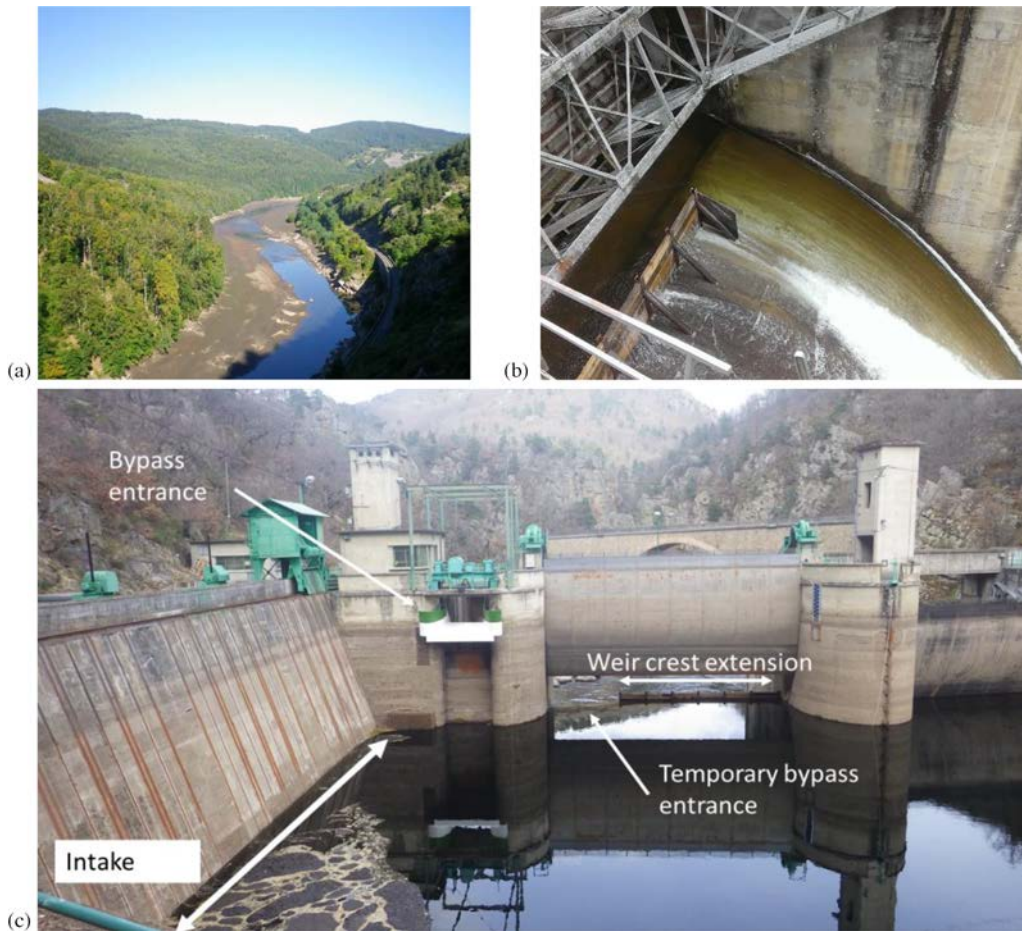
Fig. 3. Picture of upstream limit of the temporary Poutès reservoir (a). Top view of temporary bypass (b). Upstream view of intake, usual (non functional) and temporary bypass entrances (c).
