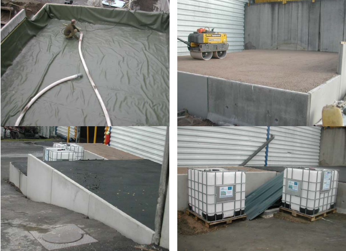
Figure 6 – Construction of the road structure for the test of lime-based binder (used in treated embankment).
