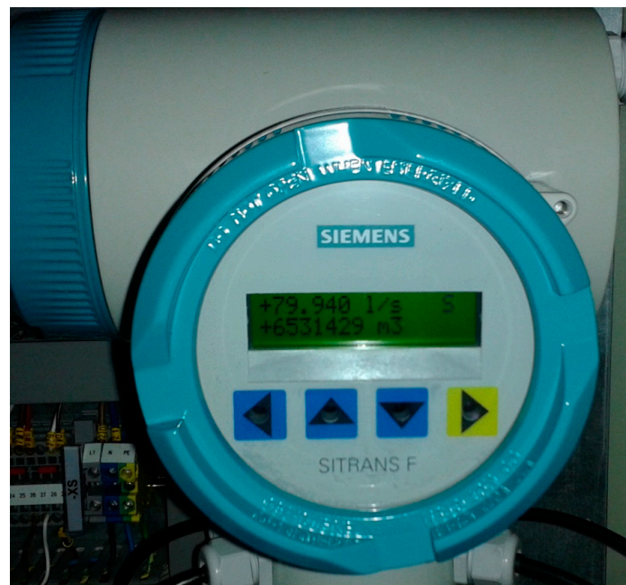
Figure 8. Ultrasonic flowmeter Siemens SITRANS F.
