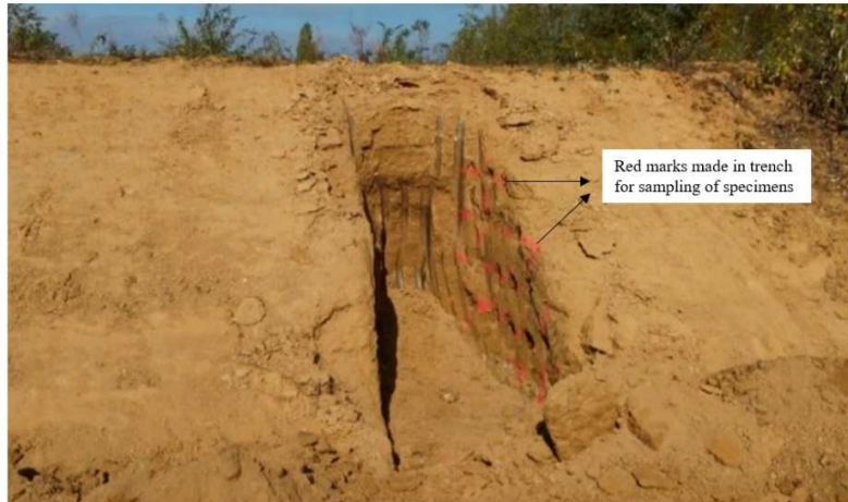
Fig. 1: Trench excavated in the lime-treated embankment (T2) for the sampling of specimens
