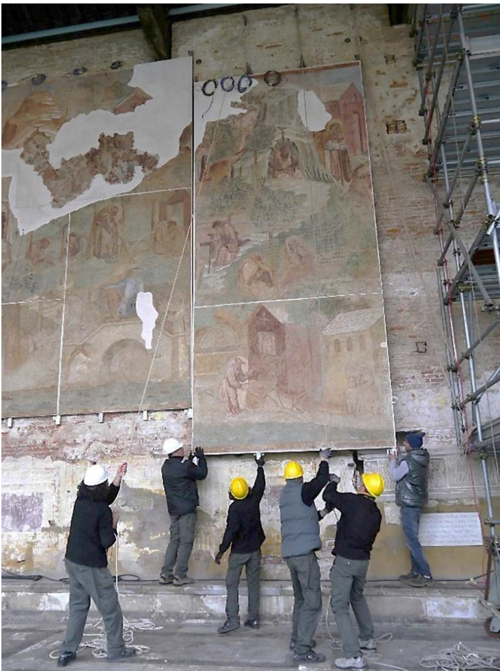
Figure 5 - Relocation of the frescoes mounted on the new heated panels onto the Camposanto Monumental Cemetery original walls.
