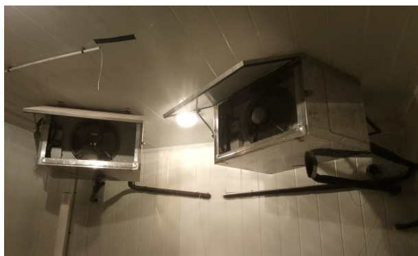
Figure 2: Photography of the two modules inside the climate chamber before the construction of the wall.
