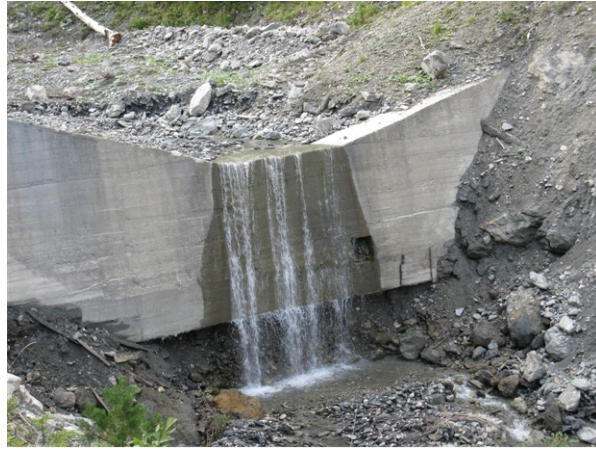
Figure 3: Scouring phenomenon downstream a check dam. Saint Antoine torrent, France, 2014. Source: ©INRAE/ETNA.
