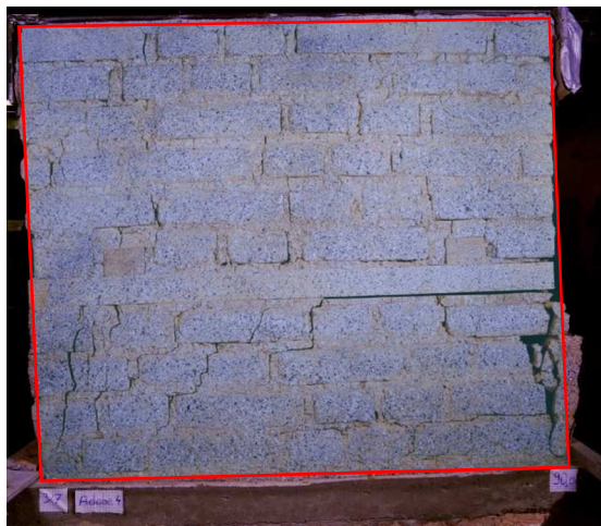
Fig. 14 Wall with timber band at 4560 seconds of loading at peak displacement towards left
