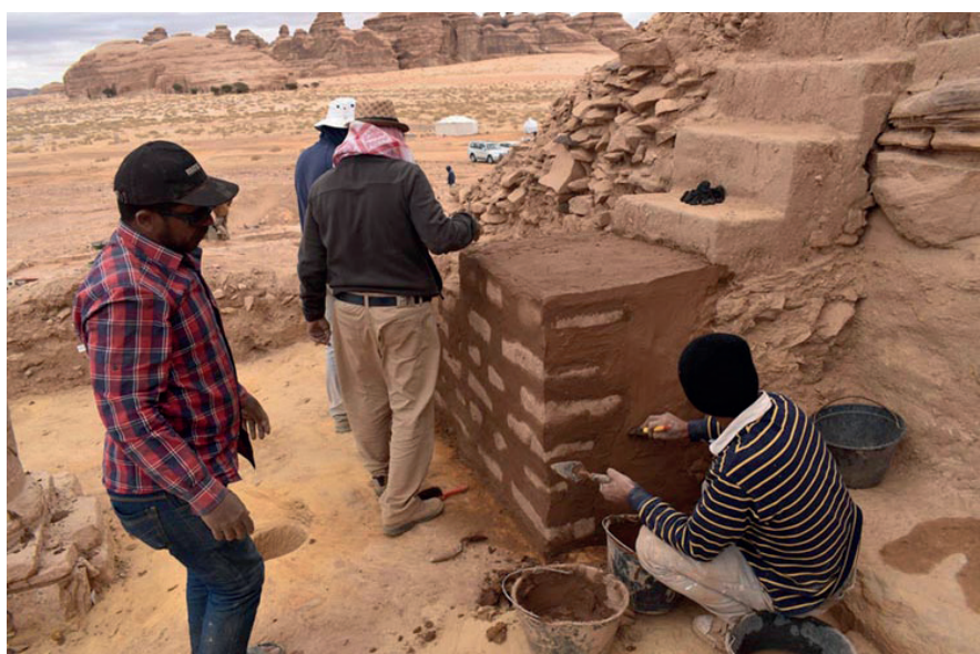
Fig. 30. Building of the staircase to secure access to the top of IGN 132.
