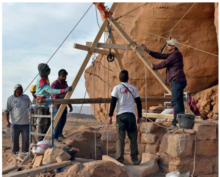
Fig. 23. Well no. 132, the two rock climbers finishing the installation of the lifting jack.
