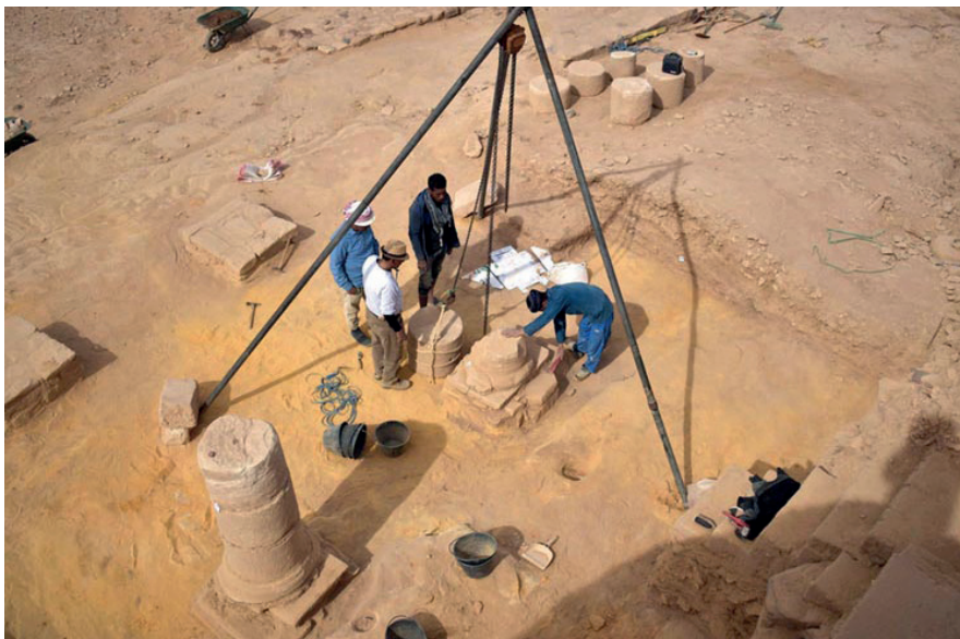
Fig. 27. The two columns in situ before the beginning of the restoration and the lifting jack.
