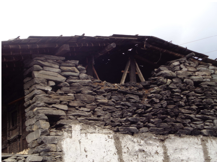
Fig. 24) Partial collapse of gable wall. Gatlang (ASF Nepal)
