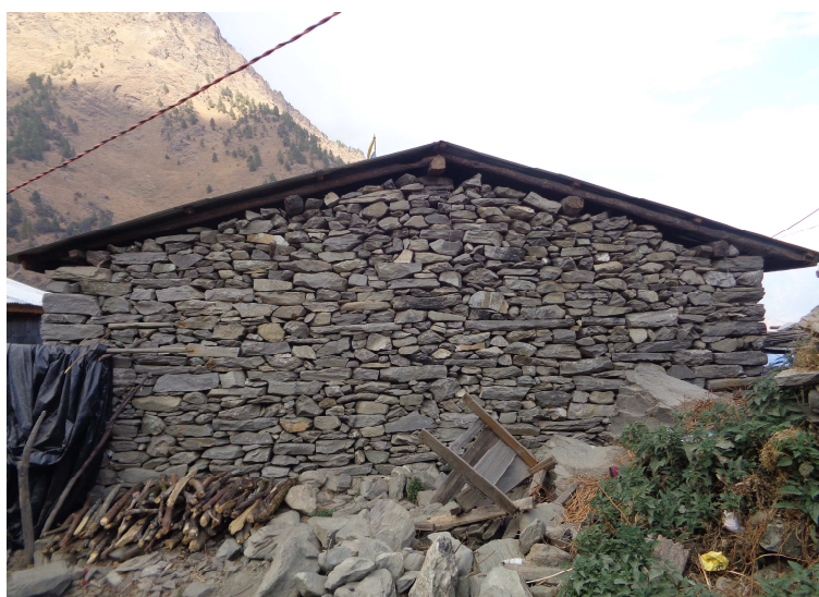
Fig. 29) partially repaired house, with addition of retrofitting component, see gable wall (CRAterre)
