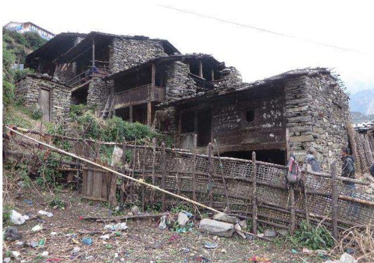
Fig. 22) Damages on gables walls on a row of Houses. Gatlang (CRAterre)
