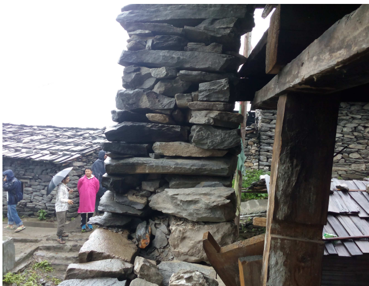
Fig. 25) Partial collapse of wall / standing wooden structure inside. Gatlang (ASF Nepal)
