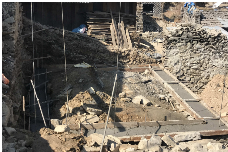
Fig.27) New house under construction beside an existing house in a row. (CRAterre)
