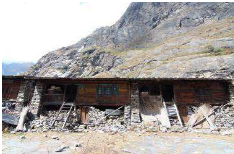
Fig.7) Row houses in Langtang Valley after the avalanches due to the 2015 Gorkha EQ.
