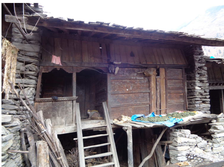
Fig. 23) Stone masonry wall distortion. Gatlang (ASF Nepal)
