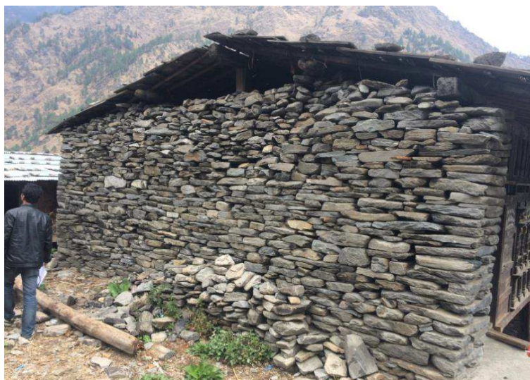
Fig. 28) partially repaired house, showing evidence of vulnerability, see gable wall (CRAterre)
