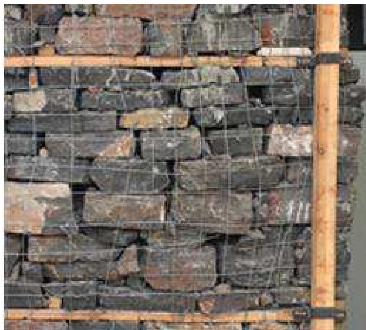
Fig. 36) Retrofitted wall sample with built-in wooden bandages with wooden posts combined with gabion wire jacketing 19
