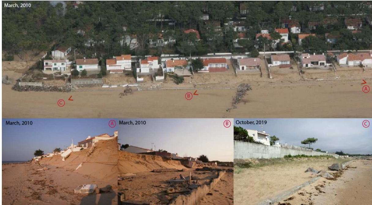
Fig. 4: The shoreline's retreat and damage on protection works in the aftermaths of Xynthia. La Tranche-sur-Mer – South of the Clémenceau beach
