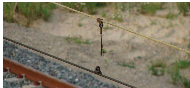
Figure 4. Dropper failure caused by fatigue.
