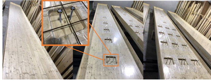
Fig. 1: Plan of beam 3 and real image of the beams before concrete casting
