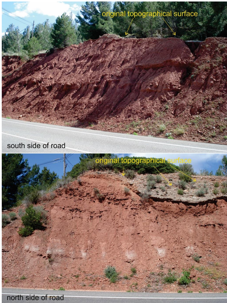
Fig. 2 Road cut slopes excavated in gypsum-cemented siltstone about 5 years after excavation. The slopes were excavated as a plane surface with a slope angle of about 60^\circ . The slopes are unstable and eroded due to solution of gypsum after excavation. The north side is less affected than the south side, likely due to more direct sunlight on the north side and the pre-failing wind direction. The protrusive banks in the south side and greyish areas in the north side are layers mainly consisting of gypsum with little silt that are slightly more resistant to solution and erosion (Road C44 near Vandellòs, Catalunya, Spain)
