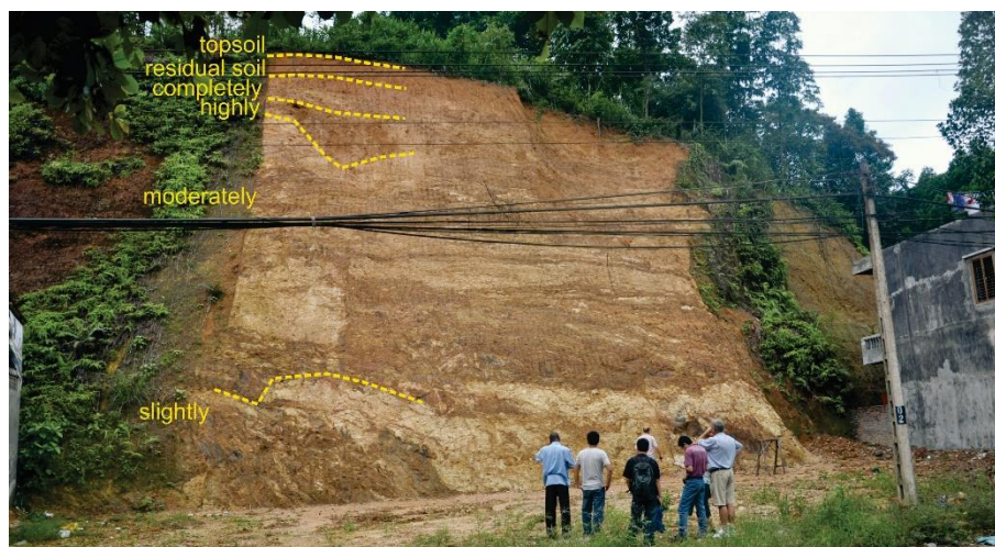
Fig. 6 Weathered cut slope in gneiss and schist in a tropical climate (Weathering grades follow Table 2 for rock masses) (Yên Bái City, Vietnam; photo courtesy D. Alkema, 2010)
