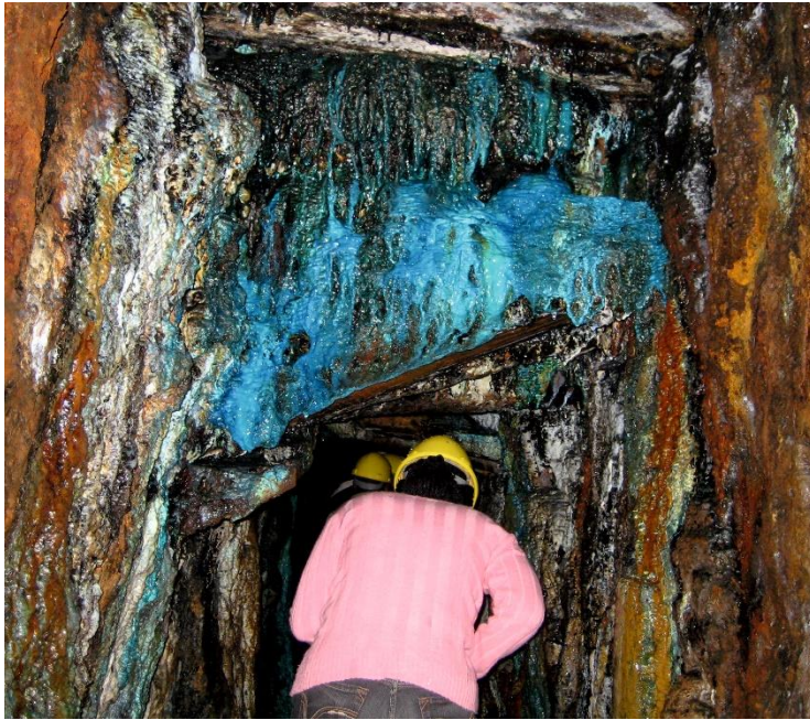
Fig. 3 Acid groundwater causing deterioration of rock mass and steel support in a mine tunnel. Oxidation of metal-sulfides by oxygen-rich percolating groundwater caused forming of sulfates and acid water. The blue and white stained areas are sulfates precipitated from seepage water (Gold, silver, copper and lead mine Rammelsberg, Goslar, Harz, Germany; photo courtesy S. Carelsen 2010)
