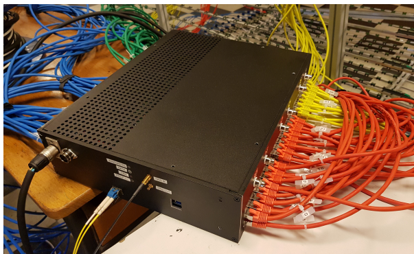
Figure 2: Photograph of the acoustic data acquisition system. The colored cables are RJ45 linking the buffer cards to acquisition system.
