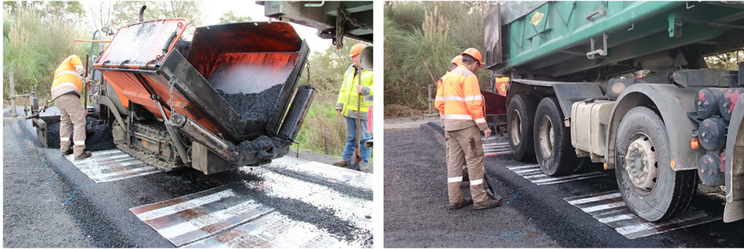
FIG. 2 Construction of the full-scale test sections and trafficking of construction equipment on the grids.
