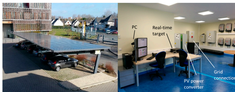
Figure 6. PV generator and control room of the technological platform.
